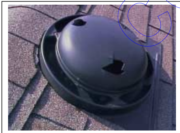
Hail damage on roof vents.
