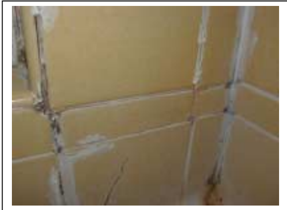
Damaged ceramic tile in master shower.
